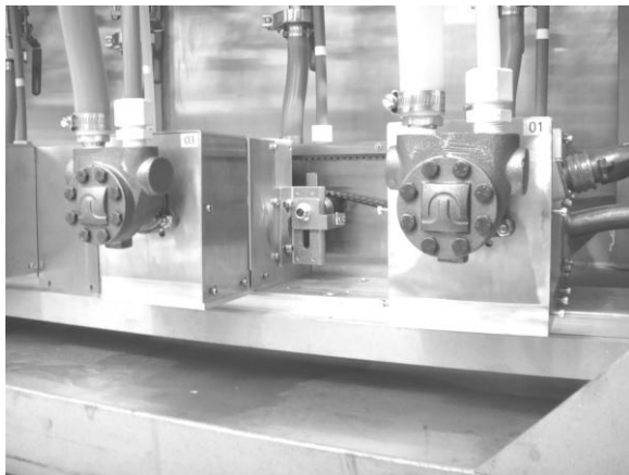
Pump Train Assembly
